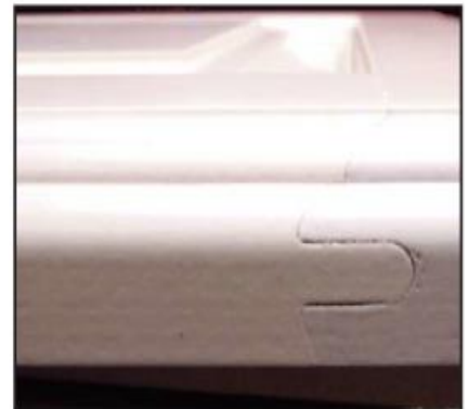
Example of door end joint separation
