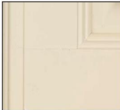
Example of door front joint separation
